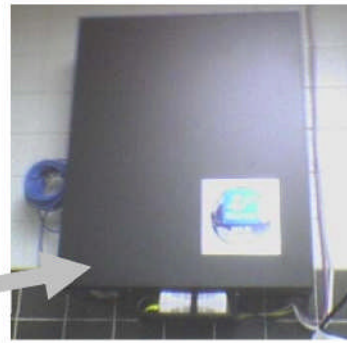
Typical Wayport Unit
